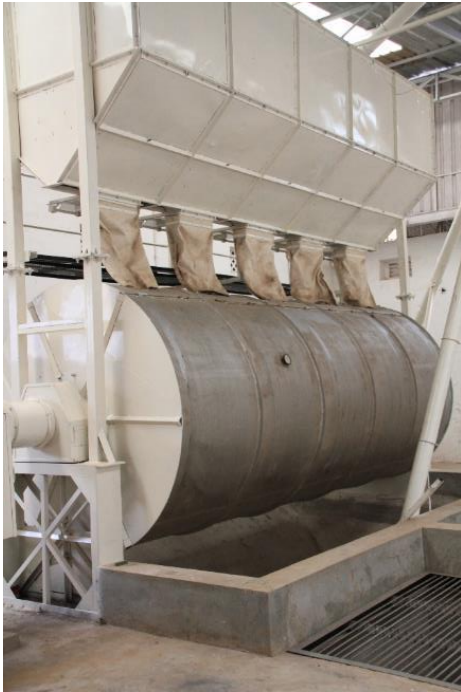
Figure 14. Mechanical drier installed at our estate
